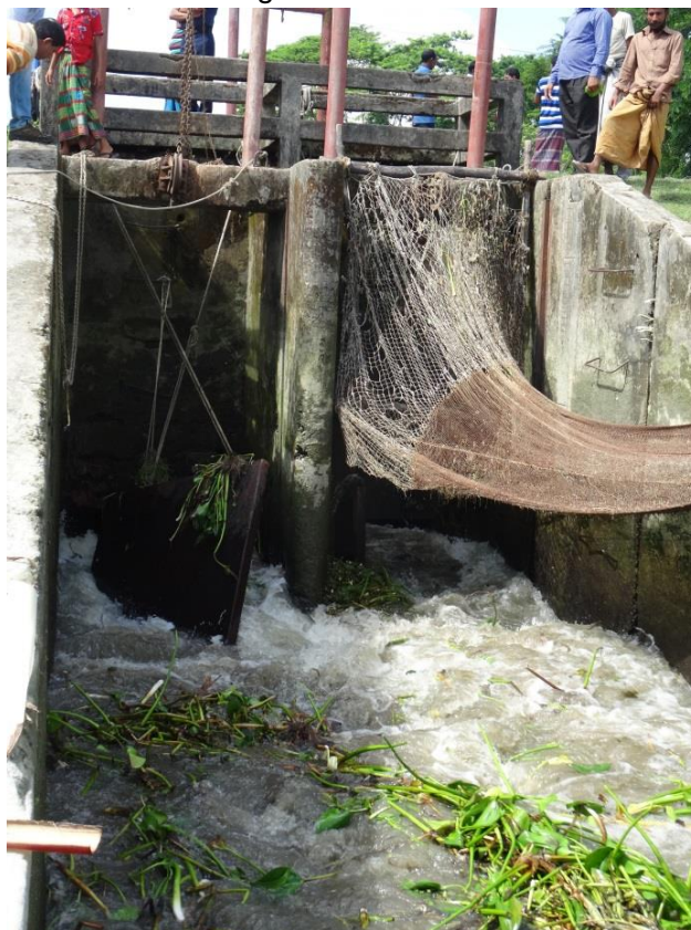
Picture 3.4: Demolished flap gate at Masurikati drainage sluice
