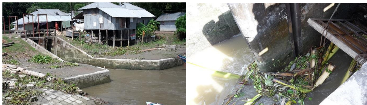
Picture 7.1 Drainage sluice Polder 43-2B with flap gates.
