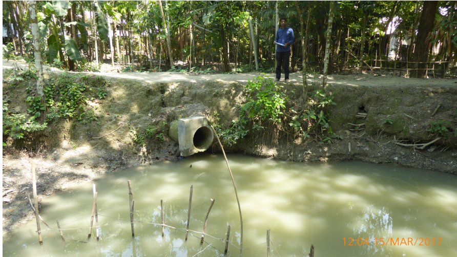
Figure 19: Erosion of an embankment section in correspondence of a pipe inlet.
