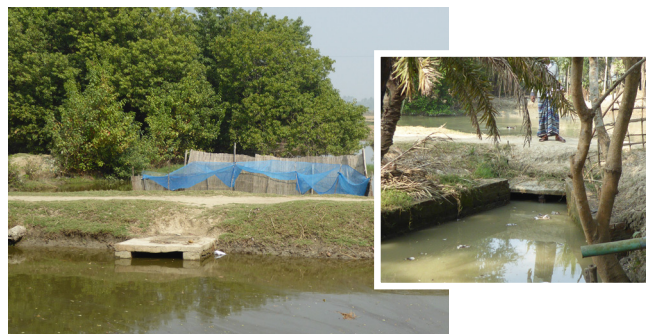
Figure 5: The box culvert upon Dangar Khal is very narrow (right). Culvert on Boyersing khal connects two khals. If Boyersing khal will be re-excavated as by plans, then the capacity of the existing culvert too low to convey the water. in March 2017, during the dry season.
