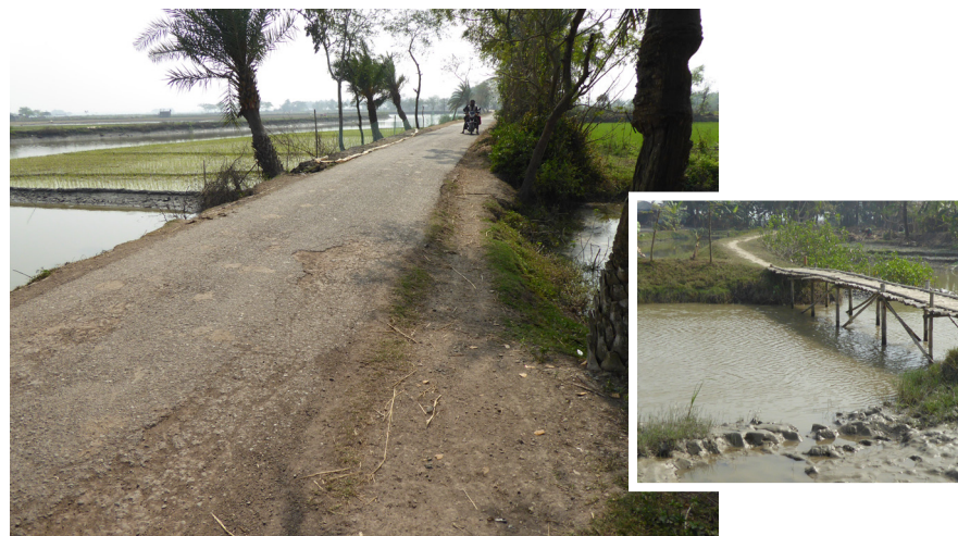
Figure 7: Main pucca Union Road cuts the Shaka Bai khal. Connectivity shall be restored by providing a large culvert on this road (left). A bridge is needed near Baloijakhi Sluice. People use a bamboo bridge to transport goods (right).
