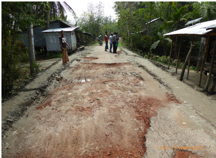
Figure 21: Poor quality embankment road.
