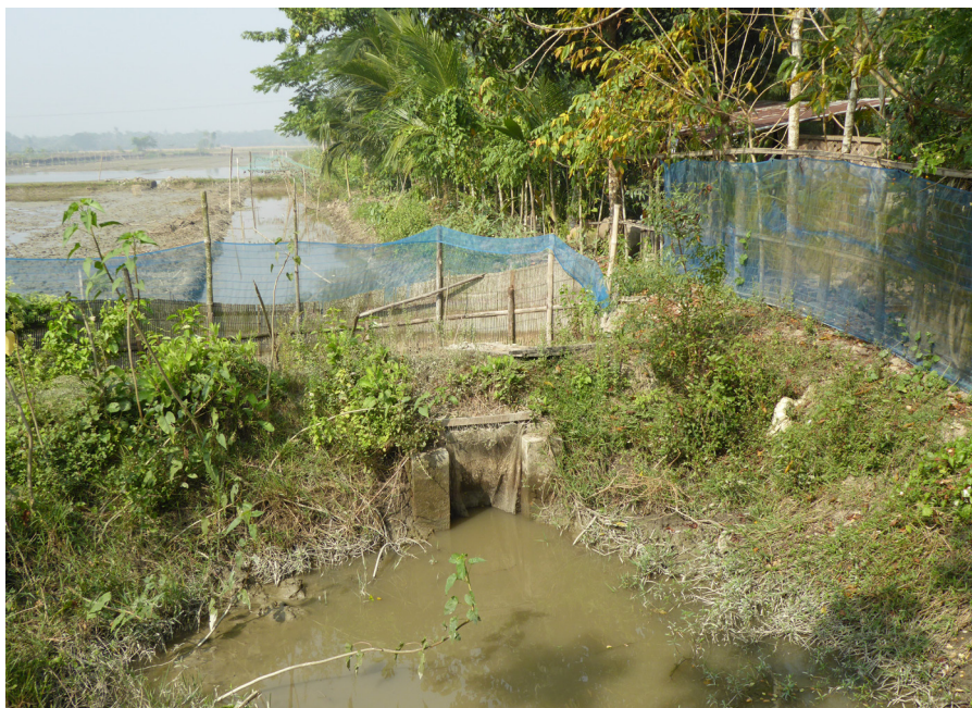
Figure 8: A fishing net in front of the opening of a culvert is encroaching on the khal system creating obstacles to the natural flowing of water and disrupting drainage connectivity.
