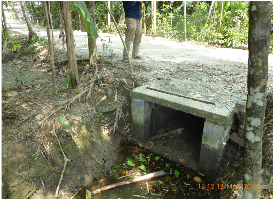
Figure 14: Gated culvert to control water flow and water levels at water crossings.
