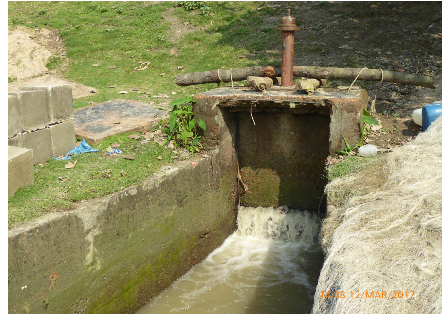
Figure 15: Defective sluice gate: this gate can neither retain water when it is needed (water losses) nor block water from entering when it is not needed (flooding).
