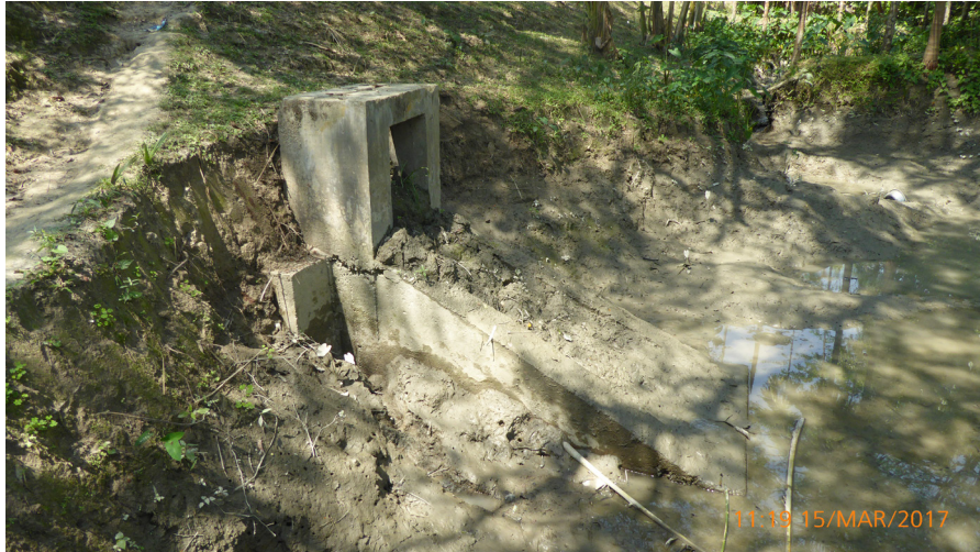
Figure 16: Inlet blocked by mud and devoid of vertical metal gate.
