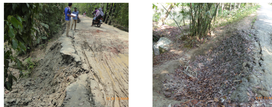
Figure 18: Two examples of erosion and degradation of embankment roads in correspondence of inlets.
