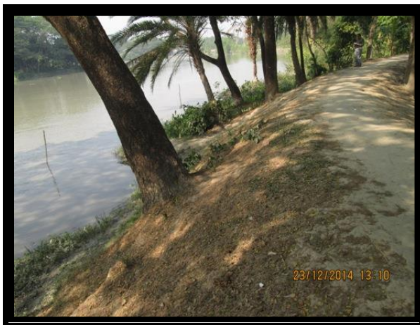
Figure1: River is at the toe of embankment at polder-43/2A
