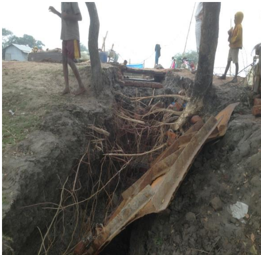
Embankment Damage due to Improper Pumping
