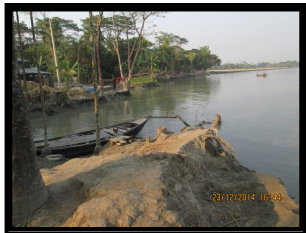
Figure1: Embankment damaged by river at polder-43/2B
