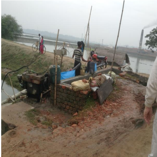
Pumps to Remove Post Monsoon Water Logging
