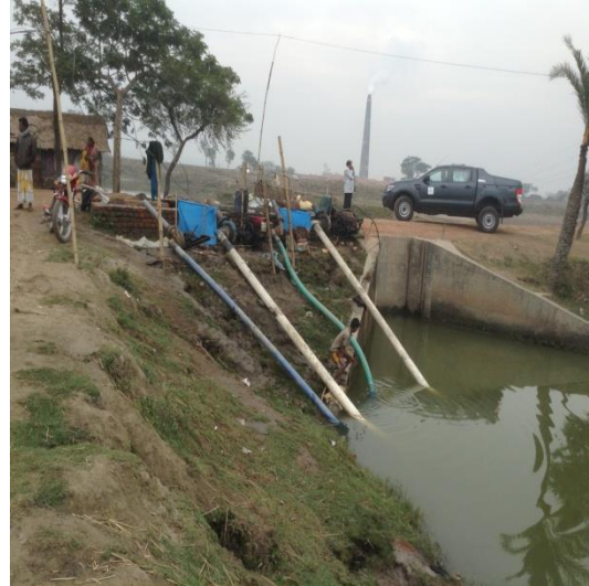
Pumps to Remove Post Monsoon Water Logging
