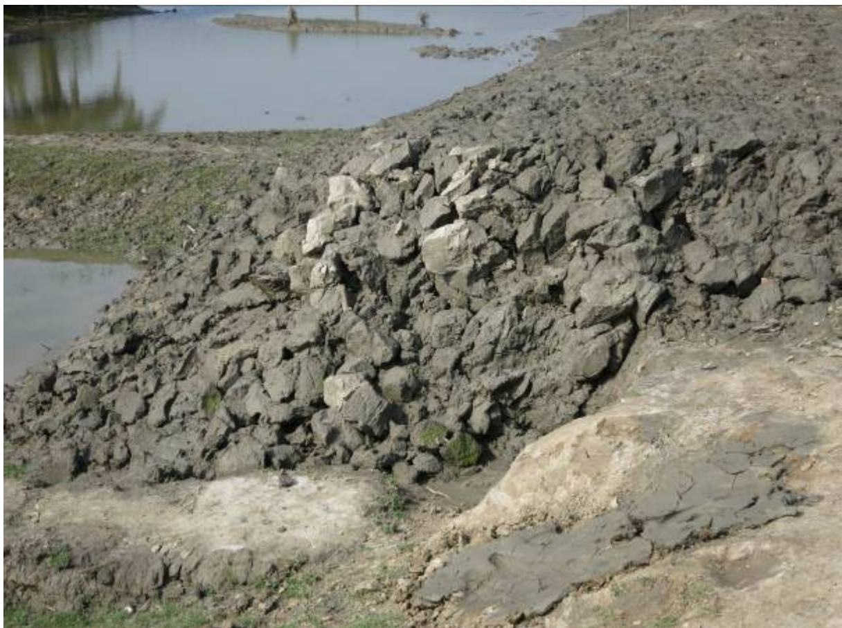
Figure 3-5 Uncompact embankment fill
