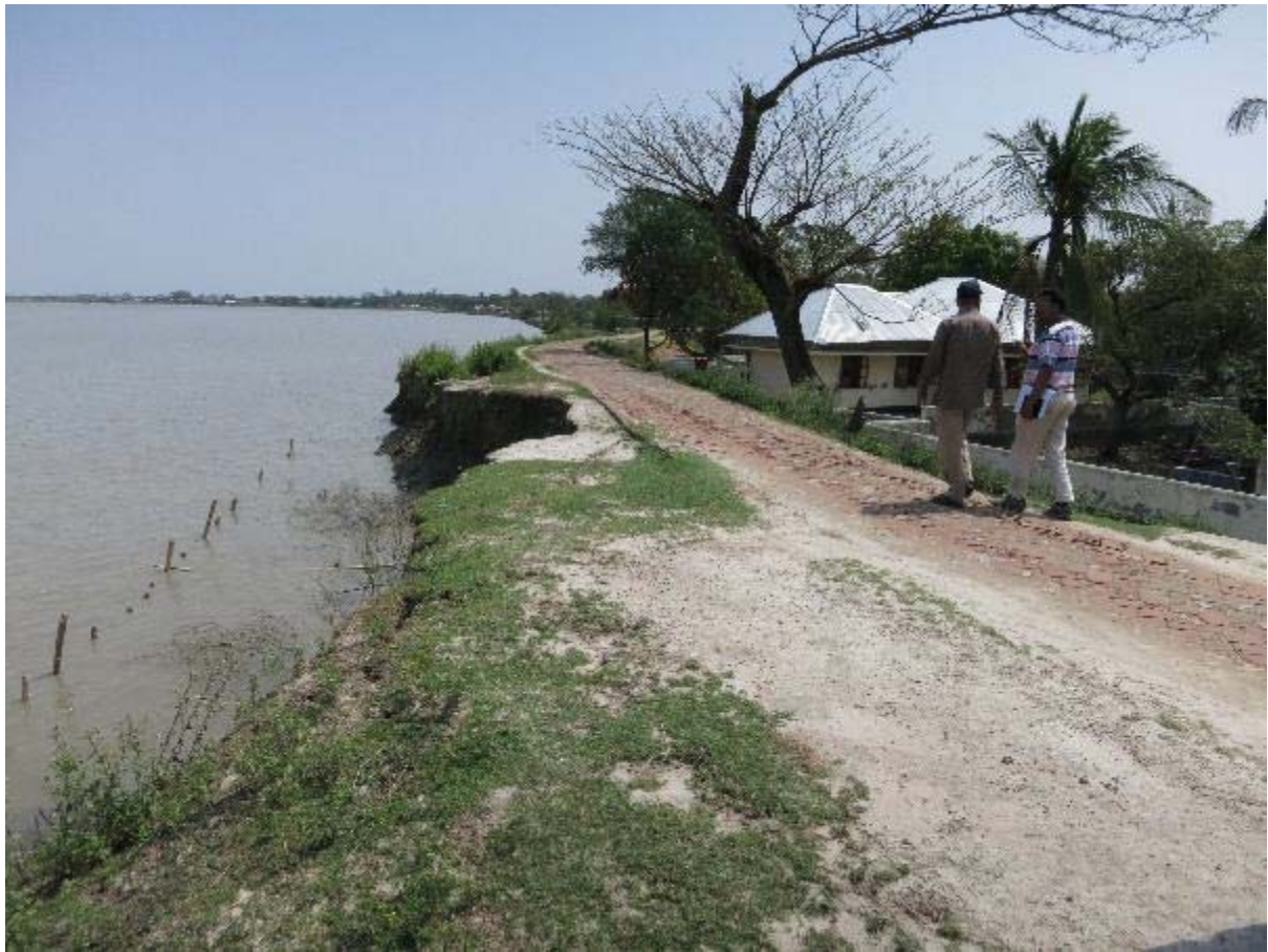
Figure 3-12 eroding riverbank with some temporary bamboo fencing
