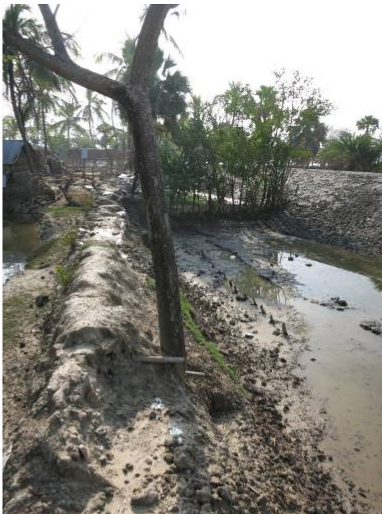
Figure 3-1 Temporary flood embankment (left hand side) and new flood embankment (background right)
