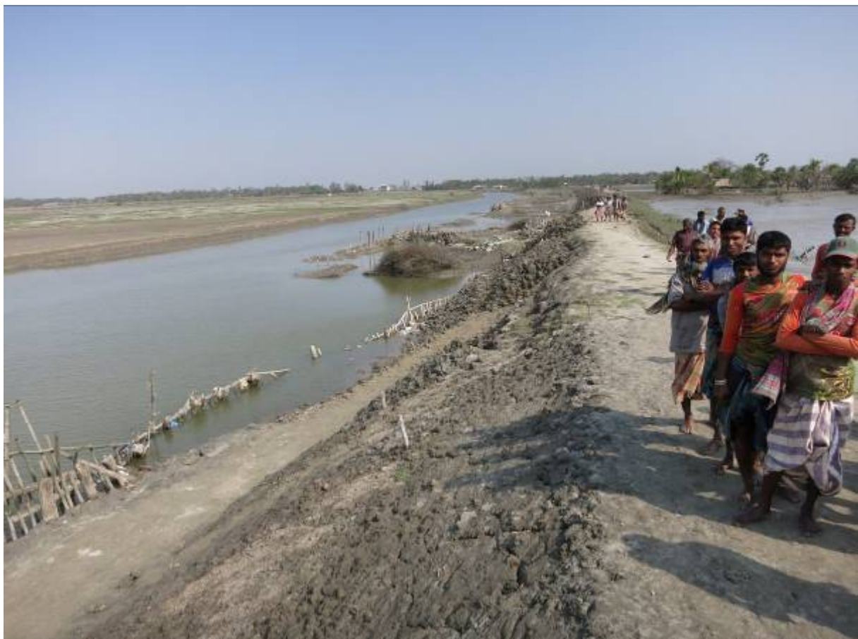
Figure 3-3 Missing berm at the main breach closure (country side view)
