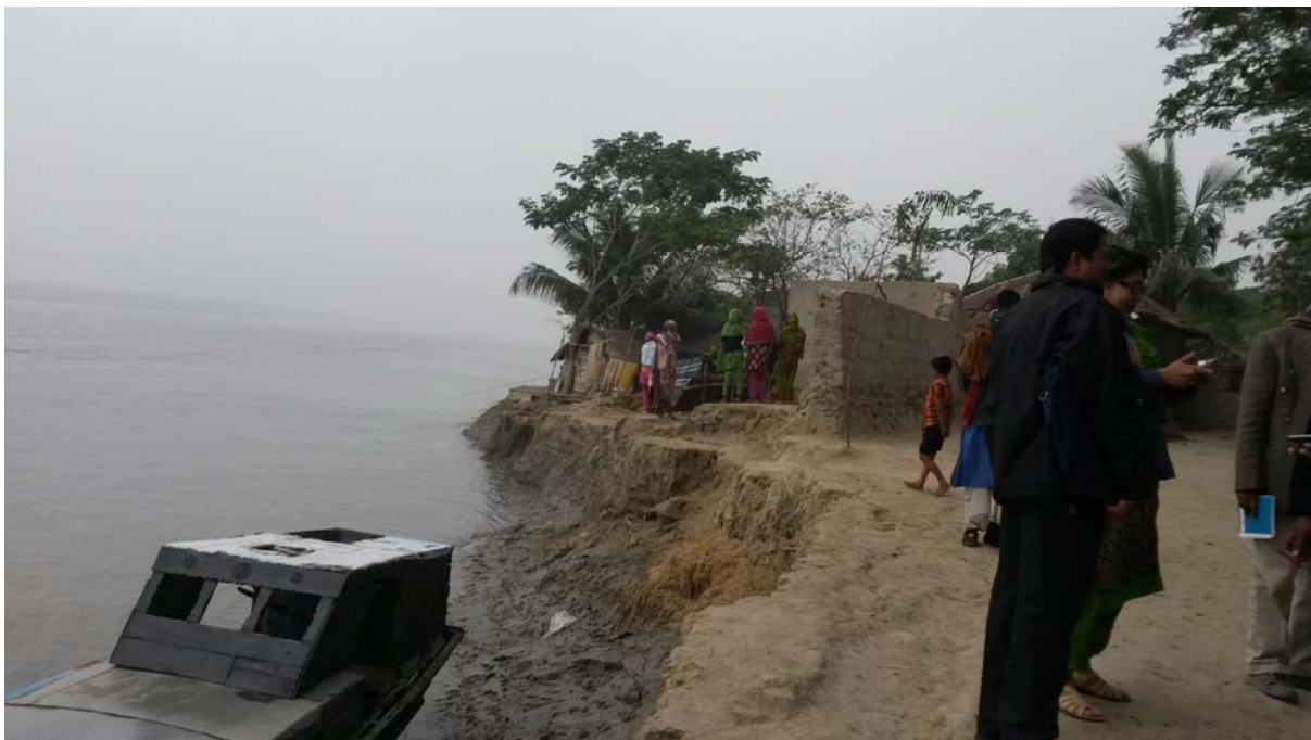
Erosion of river embankment
