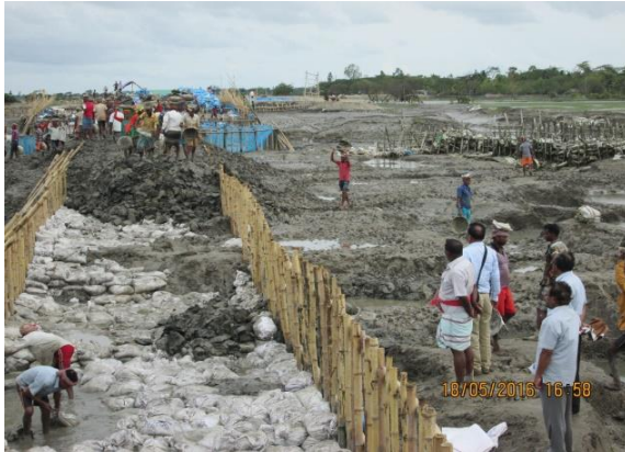
Figure-16: Closing of Second Breach with Bamboo Pins, Sand Bags and Earth (Cross Dam-2)
