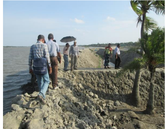
Figure-6: Temporary Ring Dike by BWDB
