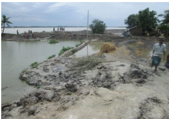
Figure-9: Vulnerable Reach Causing Breach & Channel Development
