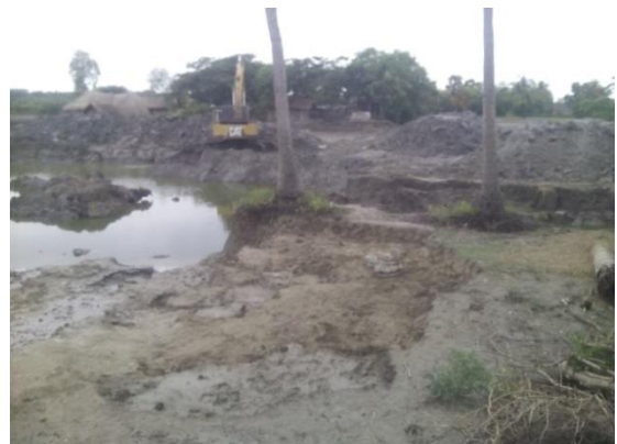
Figure-10: Vulnerable Reach Causing Breach & Channel Development
