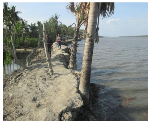
Figure-2: Continued Erosion in 2014
