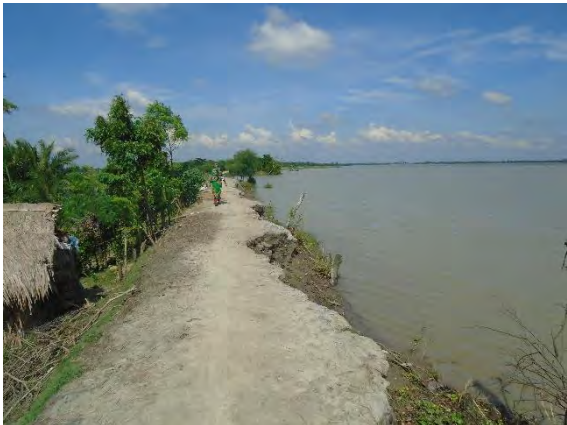
Figure: Erosion at Darun Mallik (22°35'48.00"N, 89°25'28.90"E, Dated: 01 Oct 2016)
