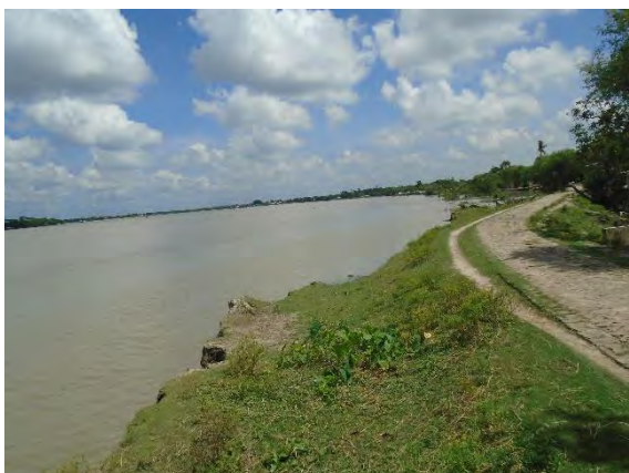
Figure: Erosion at Bigordana (22°38'32.30"N, 89°25'17.10"E, Dated: 01 Oct 2016)
