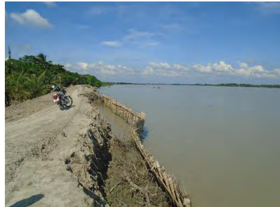
Figure: Erosion at Kalinagar (22°36'43.00"N, 89°26'27.70"E, Dated: 01 Oct 2016)
