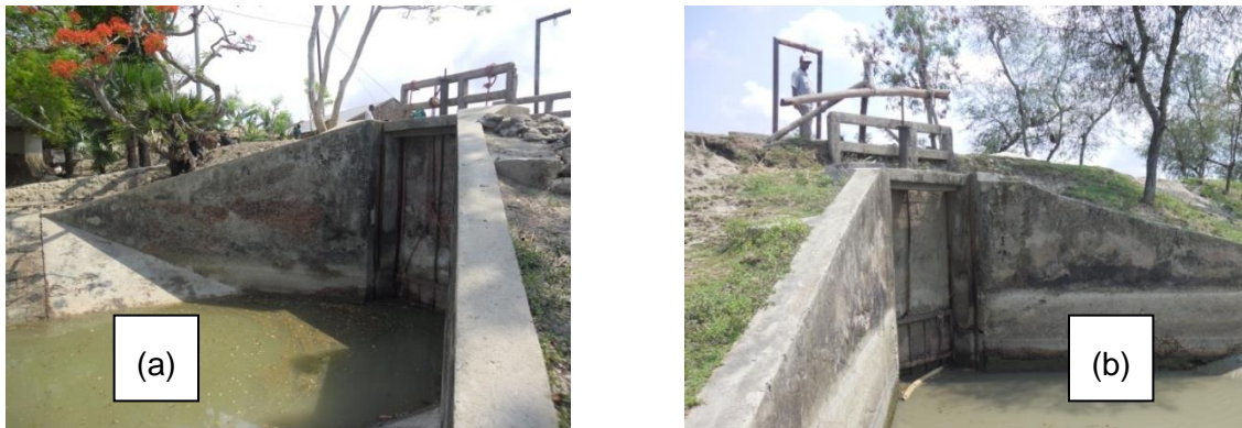
Photo 4.3: Drainage Sluice at (a) Katia Nangla Khal which needs replacement of gate and railing, (b) Moisher Danga khal which needs similar replacements
