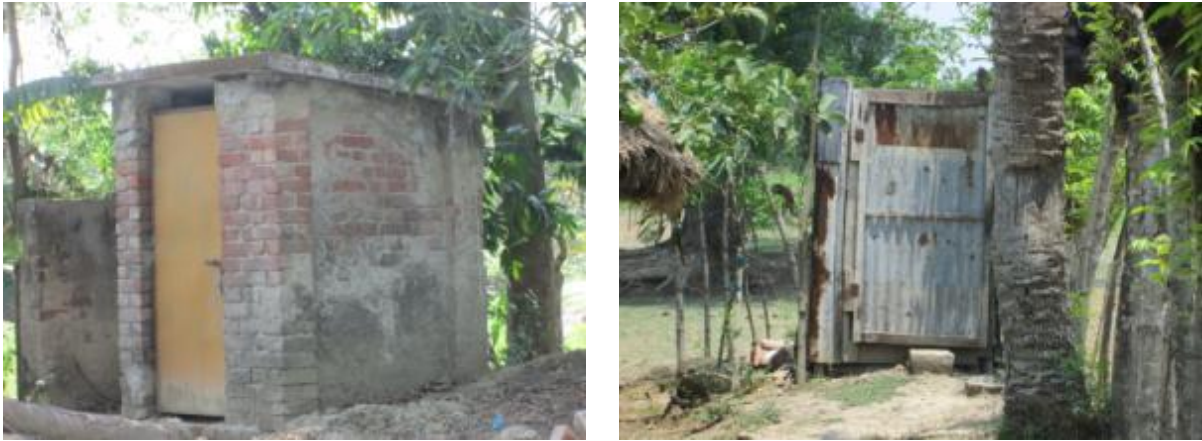
Photo 6.7: Sanitation Facility in the Polder Area
