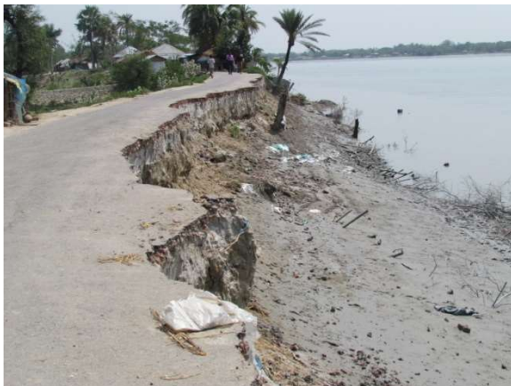
Photo 5.3: Erosion point at Baro Aria
