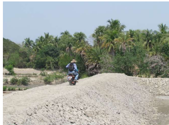
Photo 5.4: Retired embankment at the erosion hotspot at Jaliakhali
