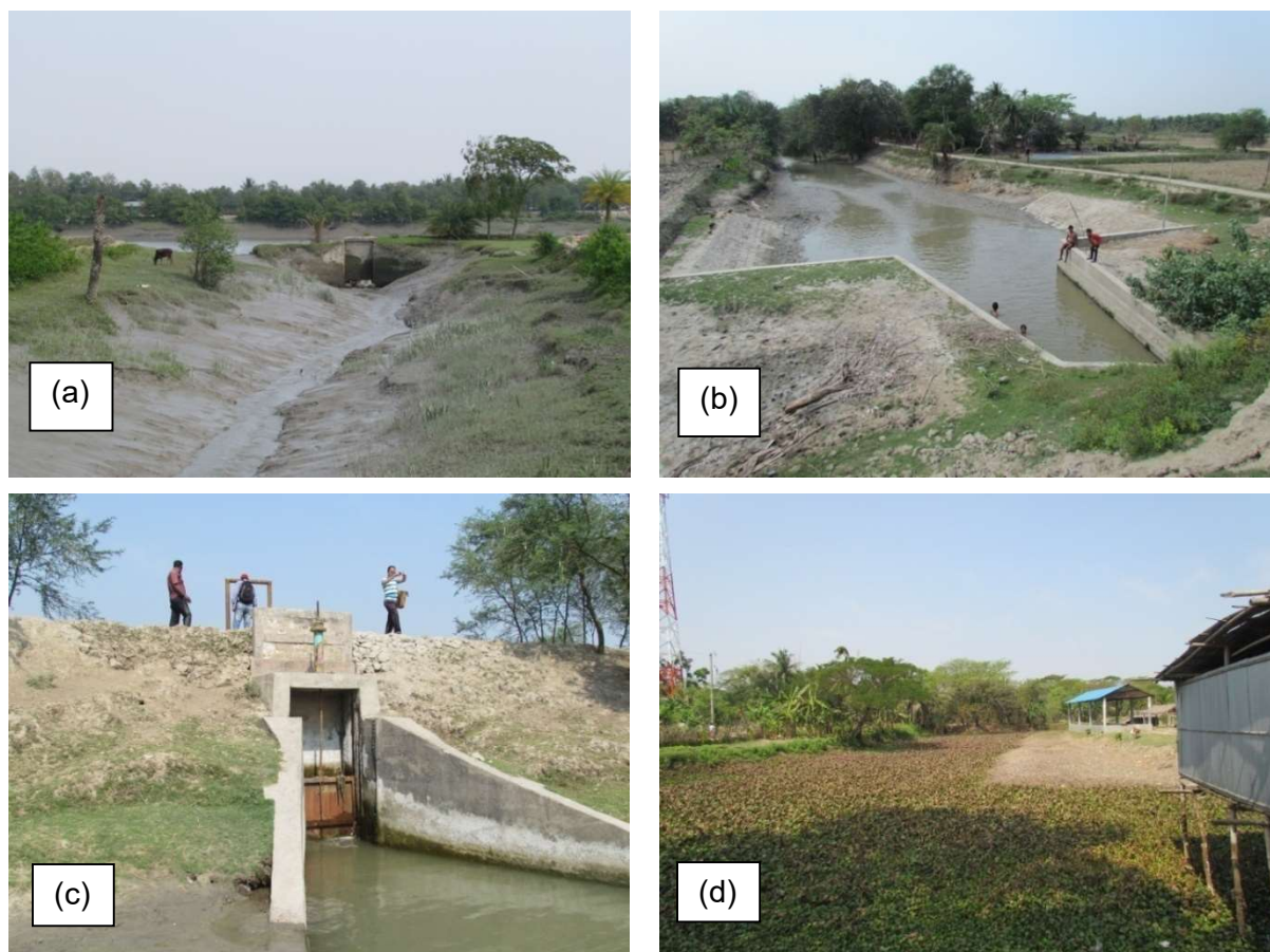
[(a) Completely broken sluice gate at Bokultala Khal, (b) Newly constructed gate inside the Bokulatola khal, (c) Sluice gate at Golaimari without a proper hoisting system, (d) Opening of Asannagar sluice covered by uncontrolled existence of water hyacinths]
