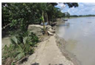
Embankment at Balaikati before it was washed away
