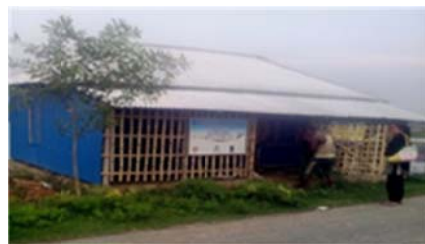
Bakultala WMG is one of those WMGs who constructed its own office without outside help. The leaders and members were united in their vision to construct their office using their own resources
