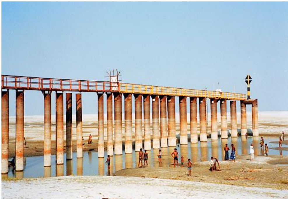
Figure 2.5. Permeable groyne test structure in the Brahmaputra-Jamuna river at Kamarjani in the dry season.
