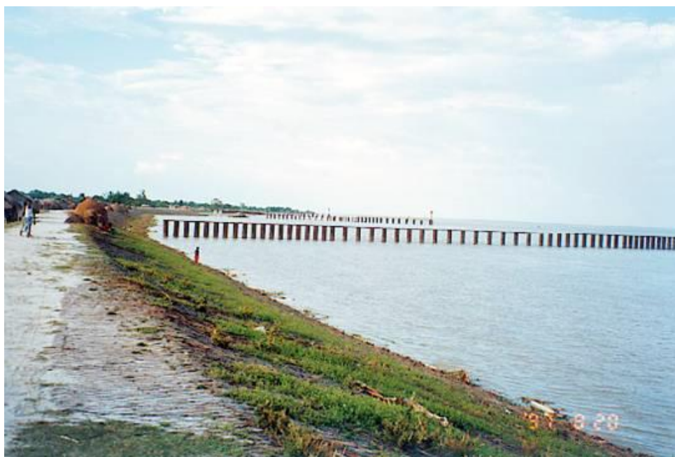
Figure 2.6. Permeable groyne test structure in the Brahmaputra-Jamuna river at Kamarjani in the wet season.
