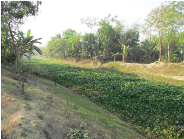
Photo 5.16 Internal canal (Silted up)
