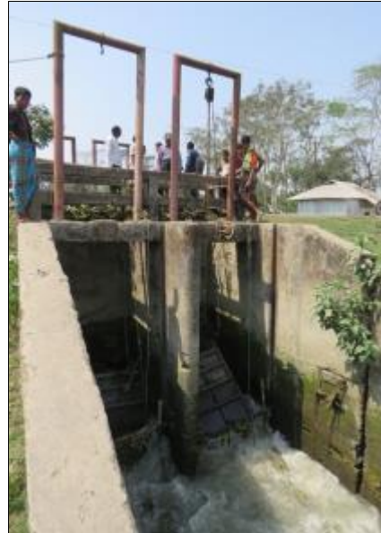
Even in the dry season the canal waters rush through the sluice gate, providing the occasional fish for the gate operator
