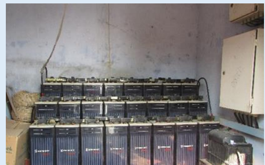
Figure: Deserted RE Electrification System
