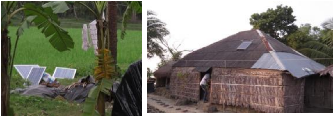
Figure 4.1.5: Application of Solar Home System
