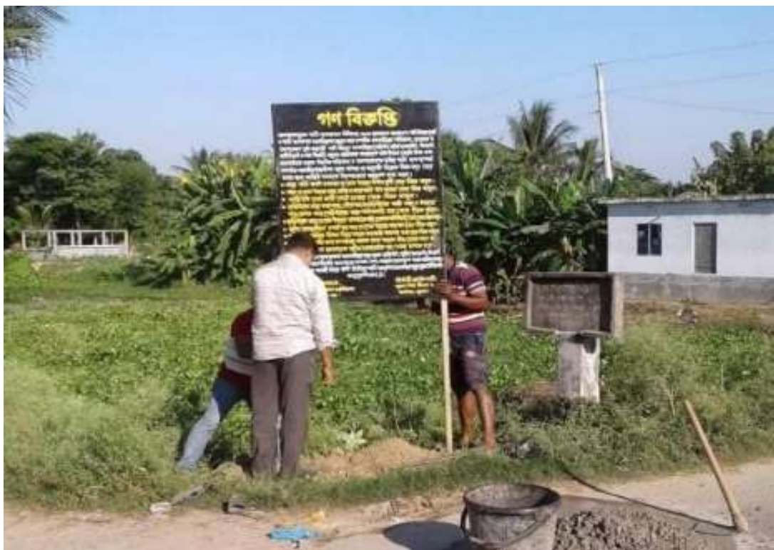
Picture 3: Catchment Committees installed warning notice by the side of the sluice gates mentioning do's and don'ts to keep water management infrastructures functional.25 , Khulna
