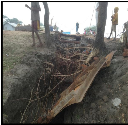
Embankment Damage due to Improper Pumping
