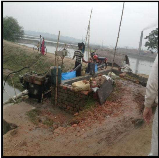
Pumps to Remove Post Monsoon Water Logging
