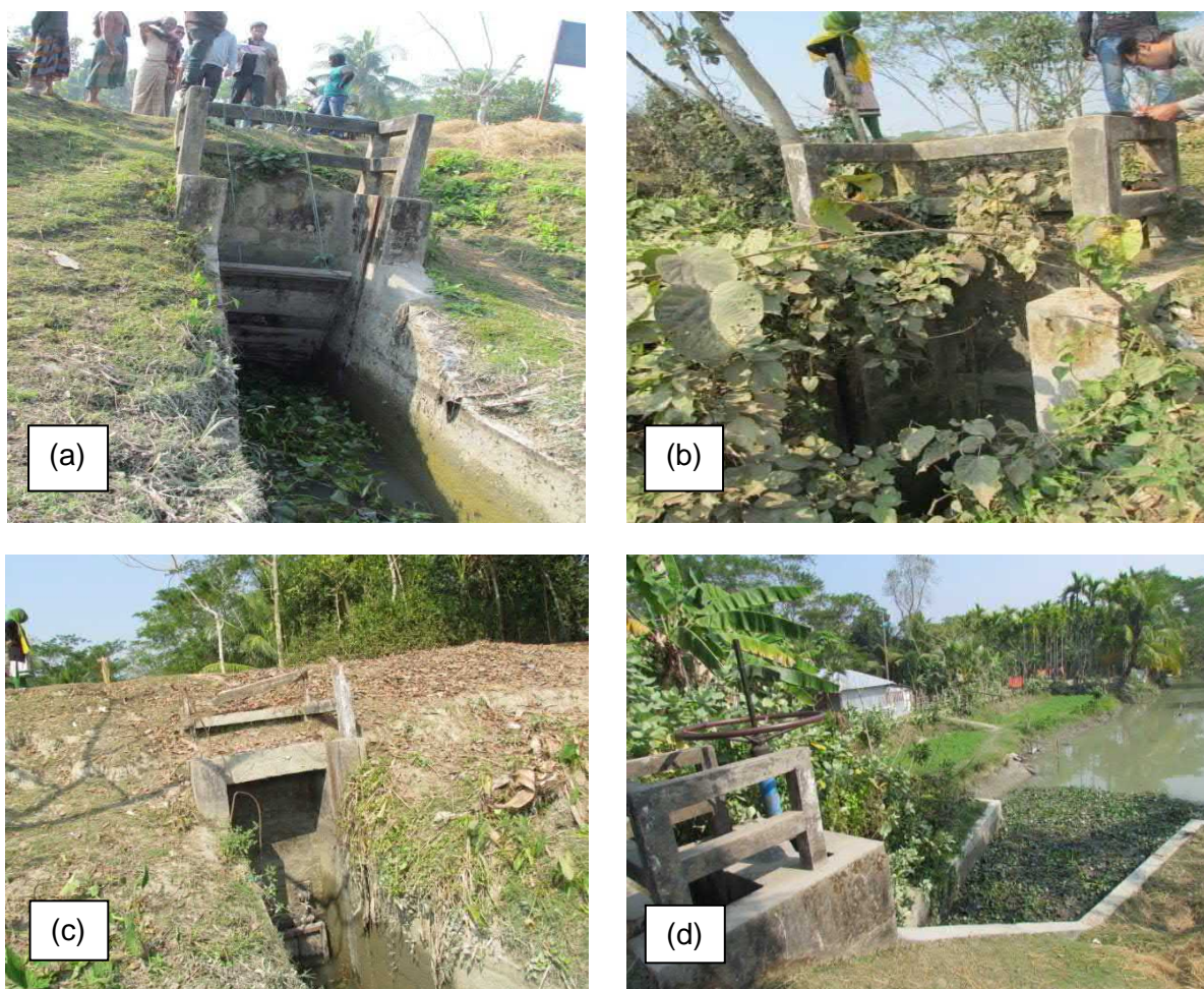
[(a) Severely damaged Dholkhali sluice requiring major repairing, (b) Non-functioning sluice gate at Katakhal, (c) Poorly maintained sluice gate at Gogonkhali, (d) Opening of Suddurbaria sluice covered by uncontrolled existence of water hyacinths]
