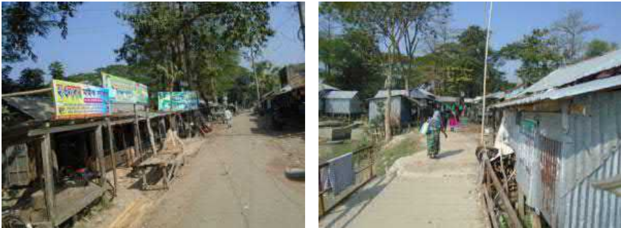
Photo 6.6: Soling and threat to damage paved road in the polder
