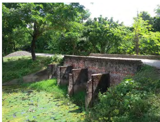
Figure: Abandon Joykhali Sluice
