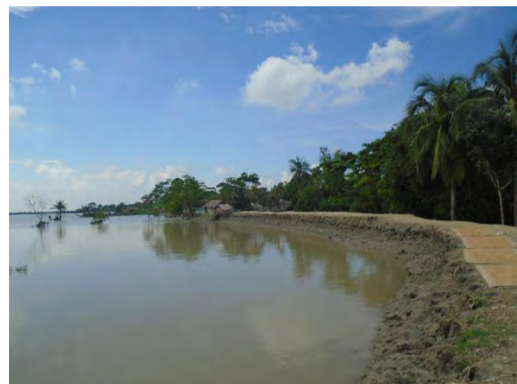
Figure: Embankment Erosion at Baro Auria
