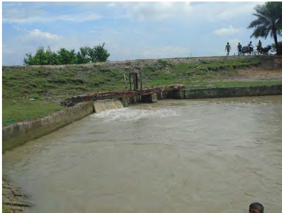
Figure: C/S of Kudlar khal Sluice (damaged)
