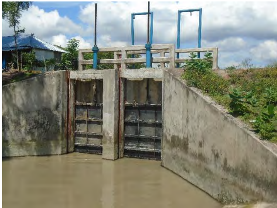
Figure: R/S of Hogolbunia Sluice
