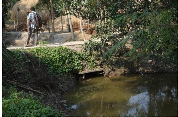
Figure 8, Footbridge blocking the main drain
