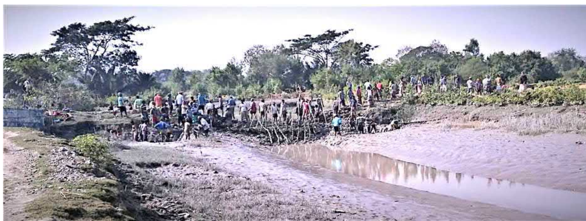
Figure 4: In Amtala sluice catchment, 8 WMGs worked together (end 2018) to excavate the outfall canal of the sluice.
