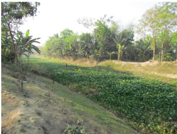
Photo 5.17 Internal canal (Silted up)
