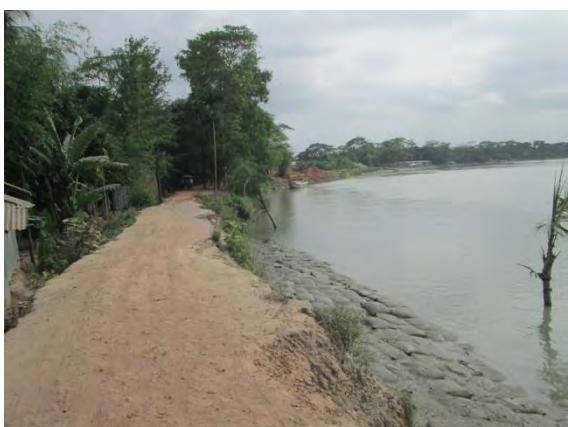
Figure: Start of River bank erosion (22° 15' 53.0" N, 90° 16' 20.3" E)
