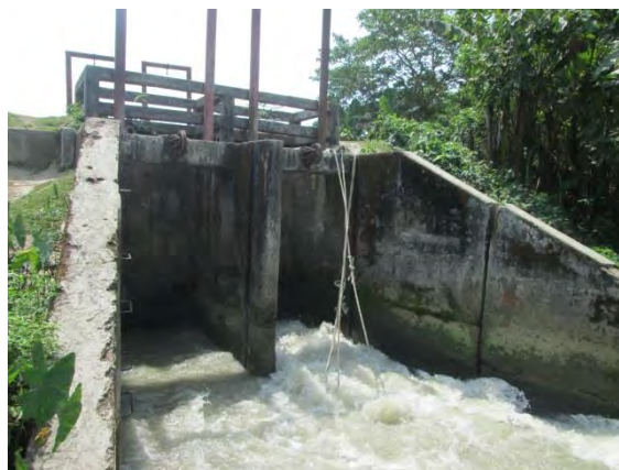
Figure: Collapsed vertical lift gate
