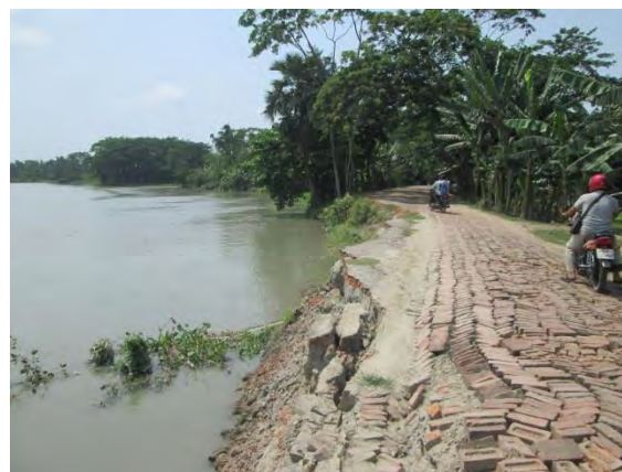
Figure: Embankment erosion at Paschim Kewabania mauza
