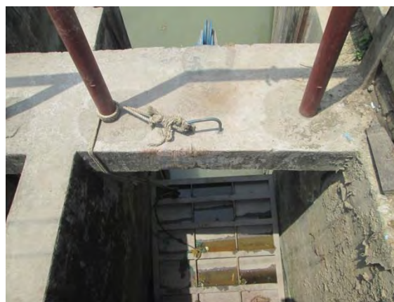
Figure: Broken flap gate of Amkhola sluice
