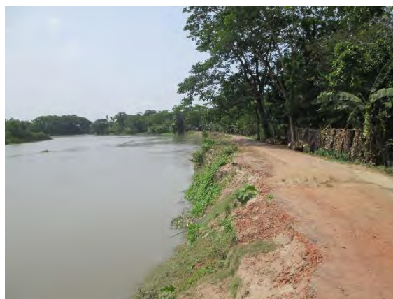
Figure: Erosion near Bashtola Outlet
